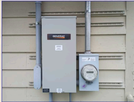
The electrical service entrance / Generator Transfer Switch
