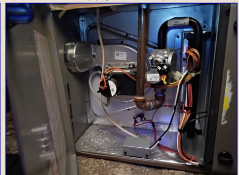
The furnace view, cover off
