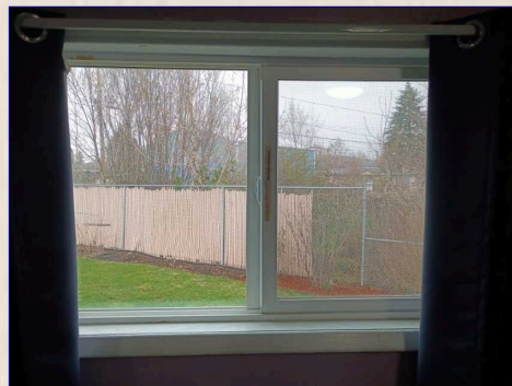
Bedroom 2 Window. Egress Restricted.
