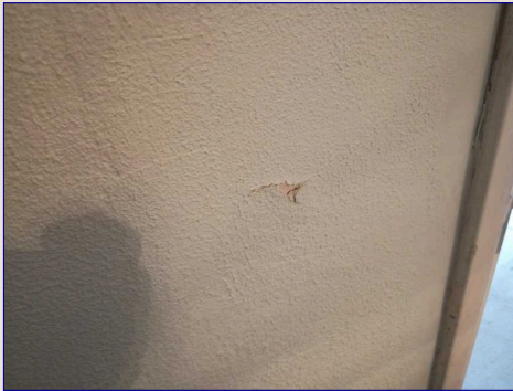
Wall Damage in Living room
