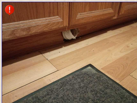
Plastic dryer vent used at the furnace.
