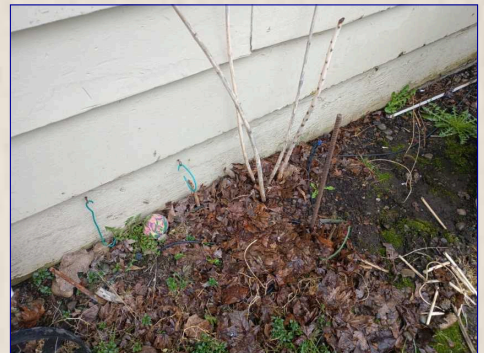
The siding is in contact with the soil.
