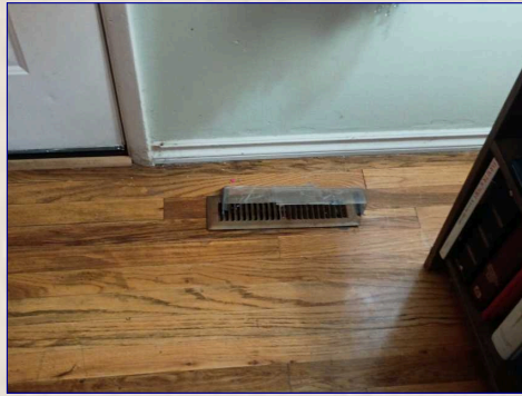
The heating vent has become damaged
