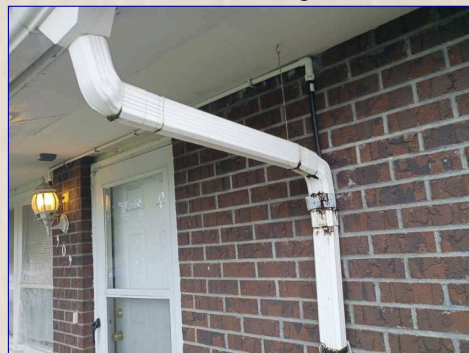
The gutter downspouts had some visible damage.
