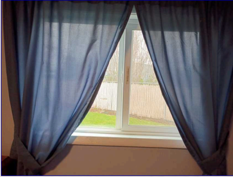
Bedroom 1 Window. Egress Restricted.
