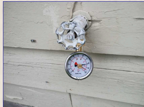
Hose bib operational.
