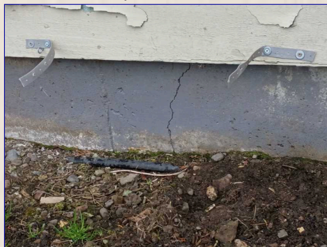
There are expected vertical cracks in the foundation.
