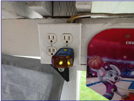
Exterior Receptacle Operating
