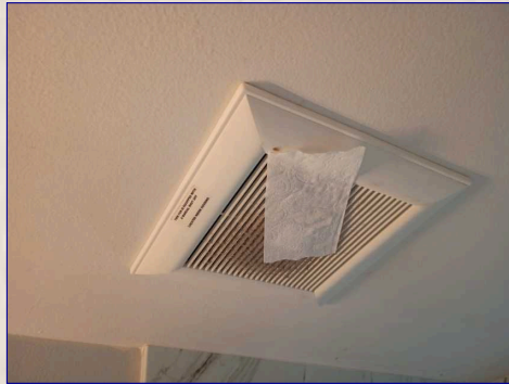
The exhaust fan operating
