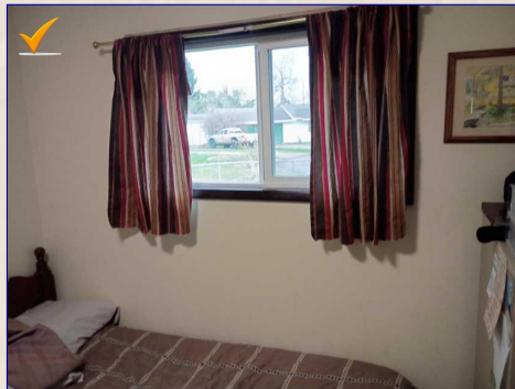
Bedroom 3 Window Egress Restricted.
