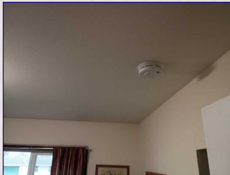
Bedroom 3 Smoke Detector
