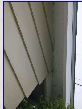
The soffit needed routine painting & maintenance.
