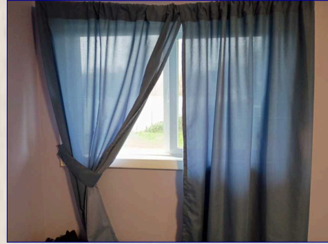
Bedroom 1 Window. Egress Restricted.
