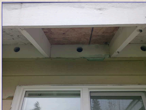
The Soffit needs routine painting maintenance.
