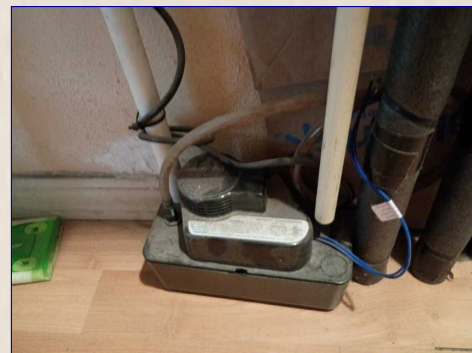
The Water Heater Condensation Pump
