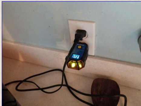
Kitchen Electrical Receptacle Operating.
