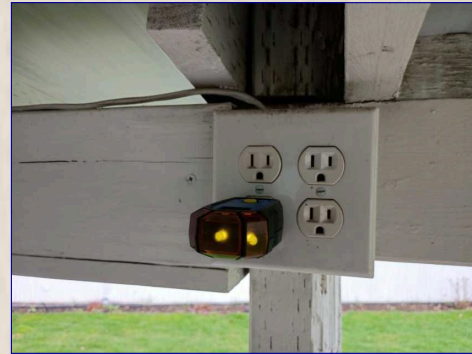
Exterior Receptacle Operating
