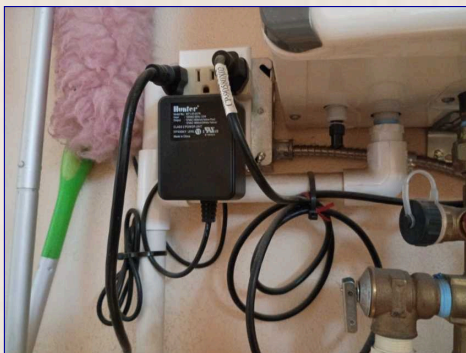
Multi Tap Electrical Receptacle at Water Heater
