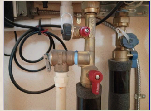
The Water Heater Water Shut Off Valve
