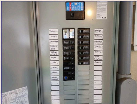
The main electrical service panel
