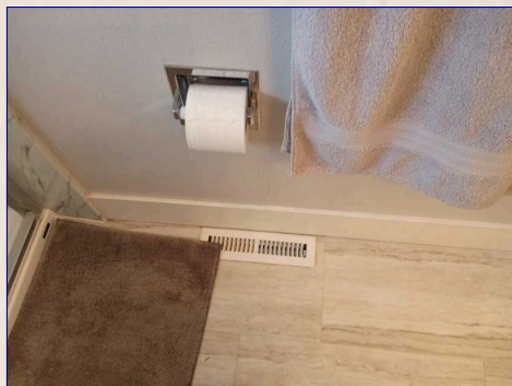
Heat source in Bathroom
