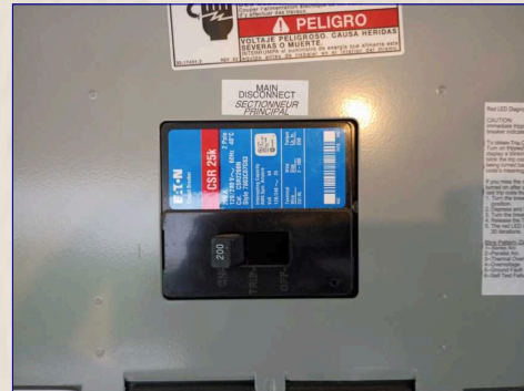
The main electrical Disconnect
