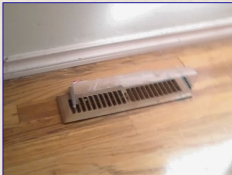
HVAC Supply Air
