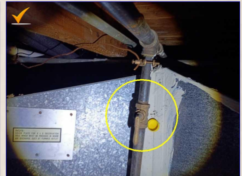
The OLD gas shutoff In line. - Recommend removing as Old Brass valves are known to leak at handle.
