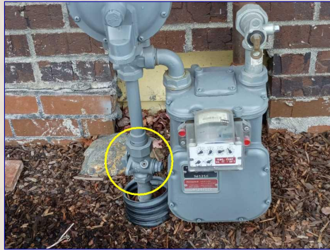
The main gas shutoff
