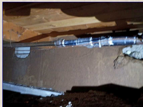
There are no wall vents in the crawl space area.
