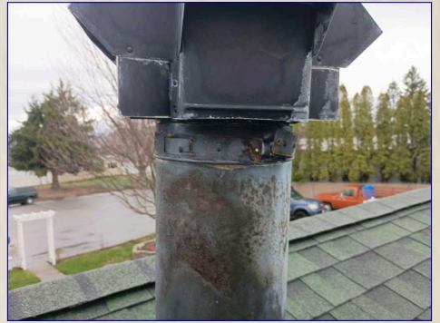
The HVAC Vent(s)
