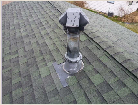
The HVAC Vent(s)
