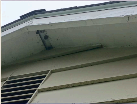
The soffit needed routine painting & maintenance.
