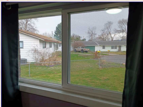
Bedroom 2 Window. Egress Restricted.
