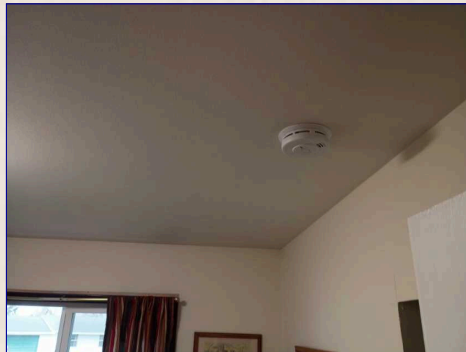
Bedroom 3 Smoke Detector
