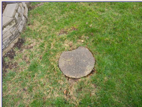
The main water shutoff
