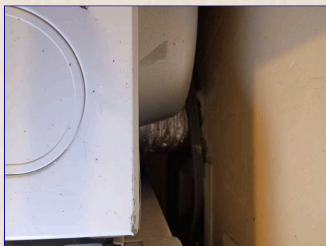
The Dryer Vent
