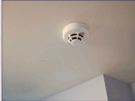
Bedroom 1 Smoke Detector
