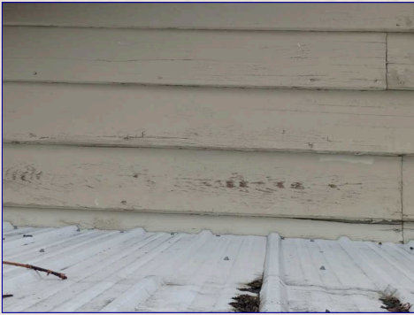
The siding needs routine repair and painting maintenance.
