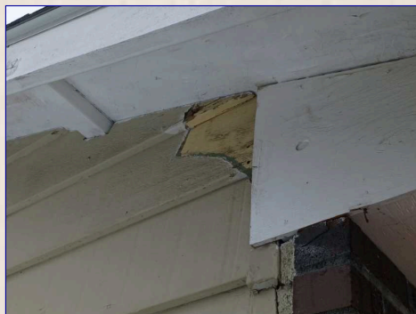
The soffit needed routine painting & maintenance.
