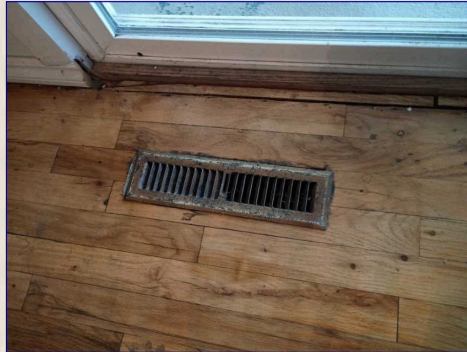
The heating vent has become damaged
