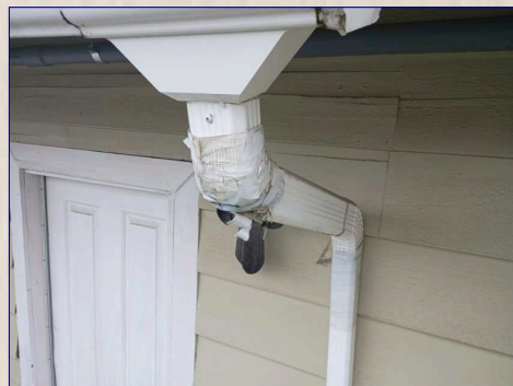
The gutter downspouts had some visible damage.
