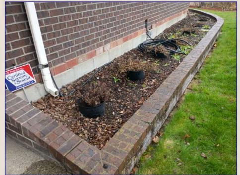
Front Flowerbed View. Downspout does not direct water far enough away from the base of the house
