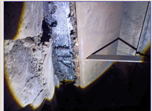
Fireplace Soot buildup
