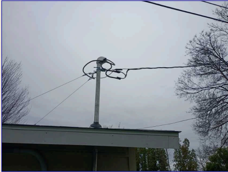
The electrical service entrance
