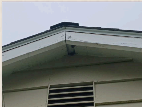
The fascia is loose, recommending a licensed contractor re-secure.
