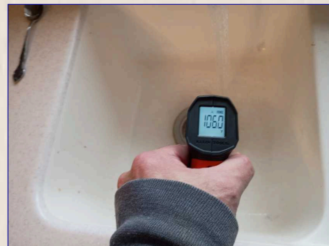
Hot Water Temperature at Kitchen sink
