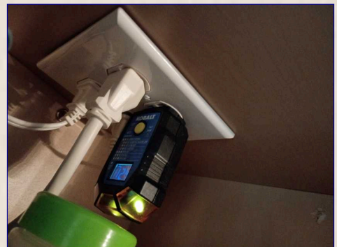
Kitchen Electrical Receptacle Operating.
