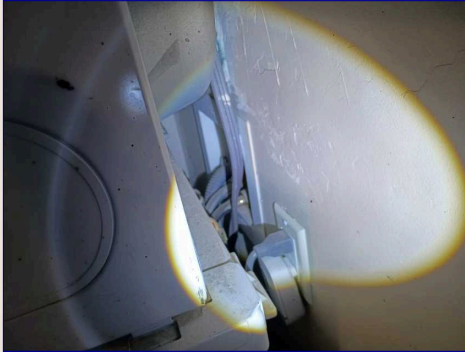
Laundry, washer hook-up view
