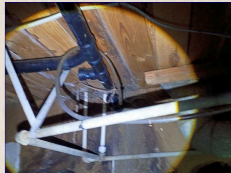
The visible drain/waste piping
