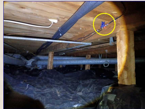
There are spliced electric wires outside of a junction box in the crawlspace. This is a safety concern. A licensed electrician should repair.
