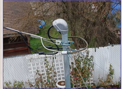
The electrical service entrance
