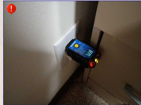
Electrical Receptacles in Bedroom 3 Wired incorrectly
