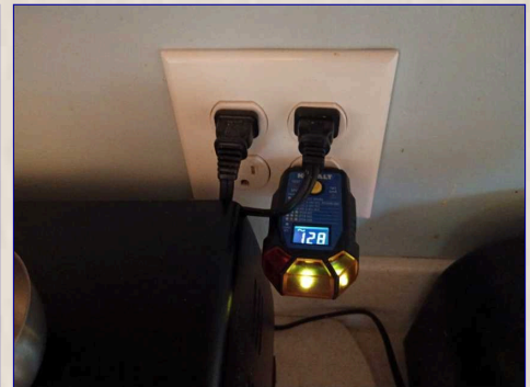
Kitchen Electrical Receptacle Operating.
