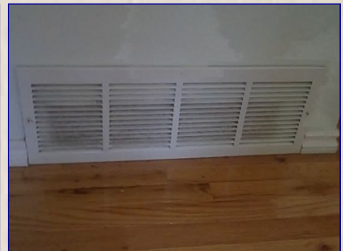
HVAC Return Air
