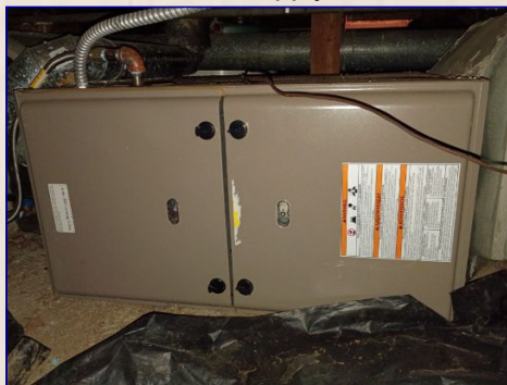
The furnace area
