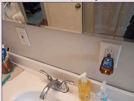
GFCI on right is master (will remove power to both)
