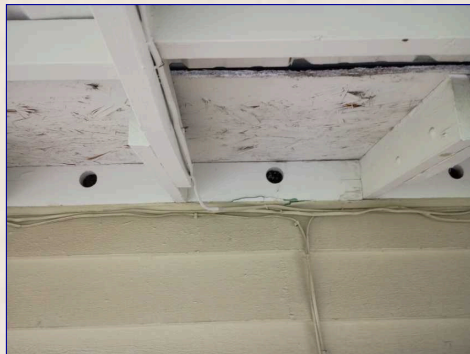
The Soffit needs routine painting maintenance.
