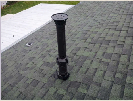
On Demand Water Heater Vent
