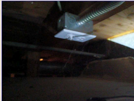
The electrical shutoff switch
