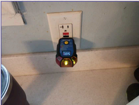
GFCI Electrical Receptacle Operating
