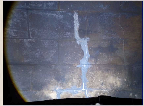
Firebrick Repair in Firebox
