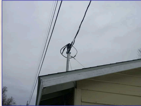
The electrical service entrance
