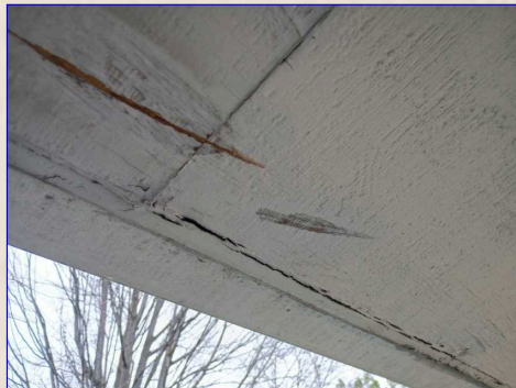
The soffit needed routine painting & maintenance.
