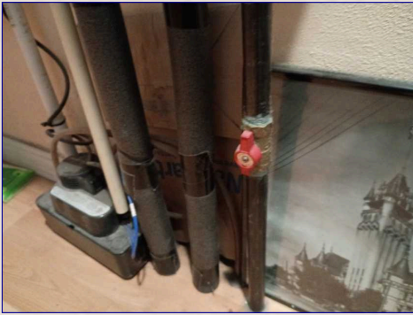
The Water Heater Gas Shut Off Valve
