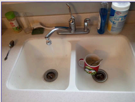
Kitchen faucet/sprayer operating
