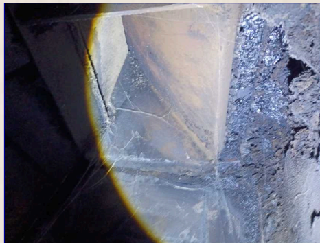
Fireplace Soot buildup
