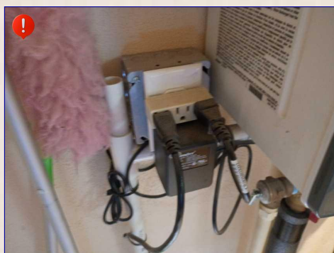
Multi Tap Electrical Receptacle
