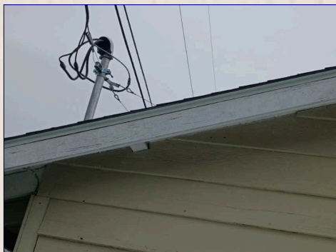
The fascia needs routine painting maintenance.
