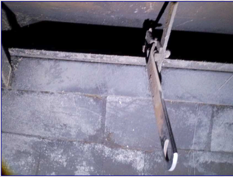
Fireplace damper is loose and does not stay closed securely.
