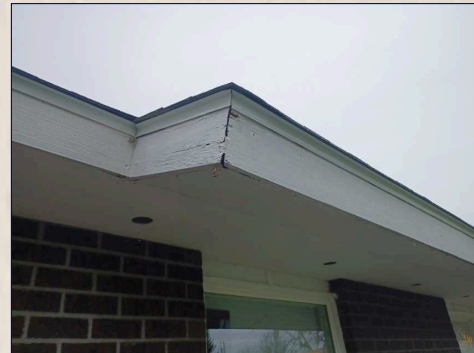
Roof Flashing. Soffit / Fascia needs maintenance
