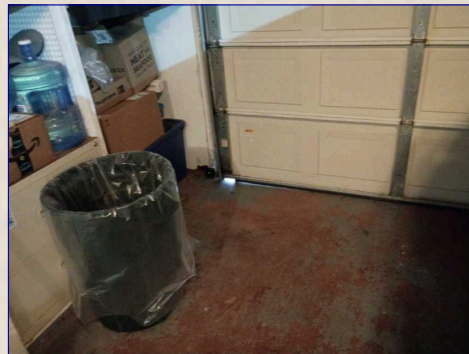
The garage door weatherstripping is missing or damaged.
