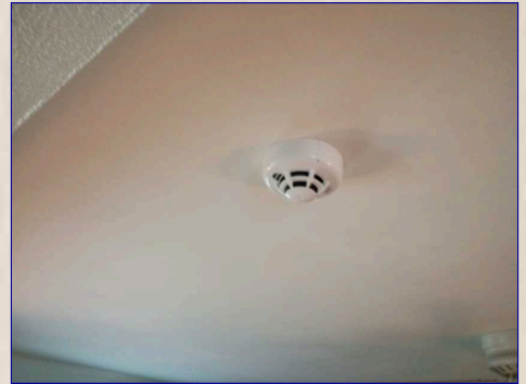
Living Room Smoke Detector
