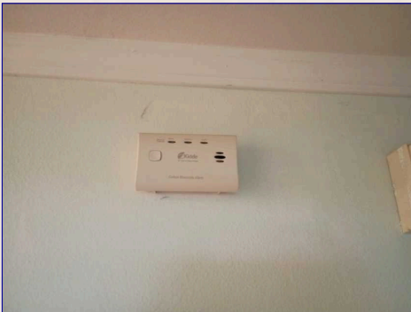
CO Detector in Main Hallway
