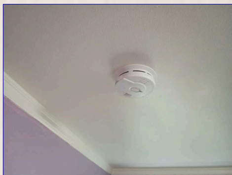
Bedroom 2 Smoke Alarm
