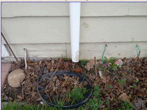
The gutter downspouts don't direct water far enough away from the house.
