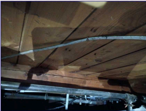
Cloth covered Romex Branch Wiring
