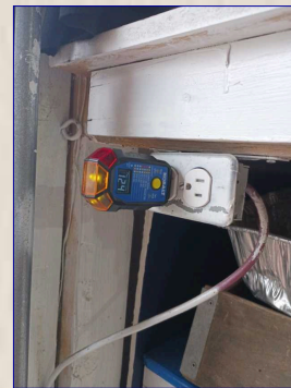
Electrical Receptacle Operating
