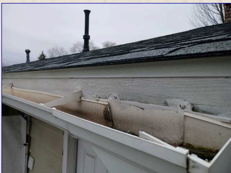
The gutters are dirty. Recommend cleaning the gutters
