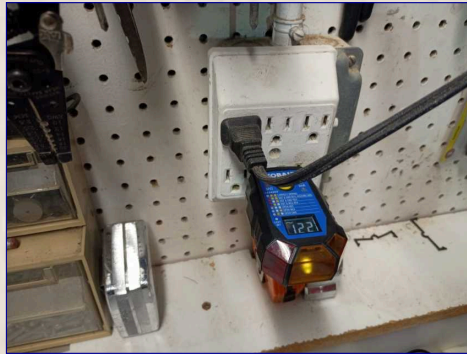
Electrical Receptacle Operating
