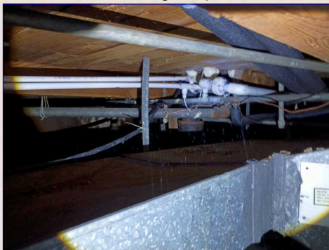
The visible drain/waste piping
