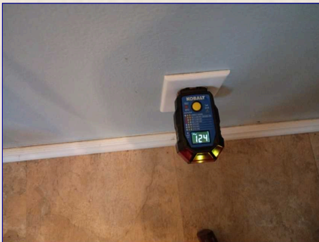
Kitchen Electrical Receptacle Operating.
