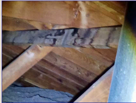
There are Moisture stained rafters/trusses in the attic. No Active moisture detected, Recommend Monitoring area above refrigerator in Kitchen
