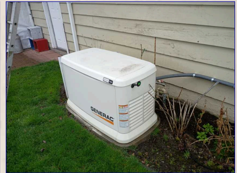
Natural Gas Generac Generator
