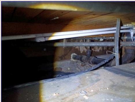
Main Plumbing Drain
