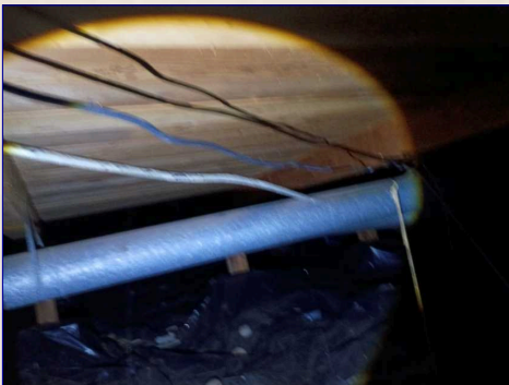
No visible insulation was noted in the crawlspace
