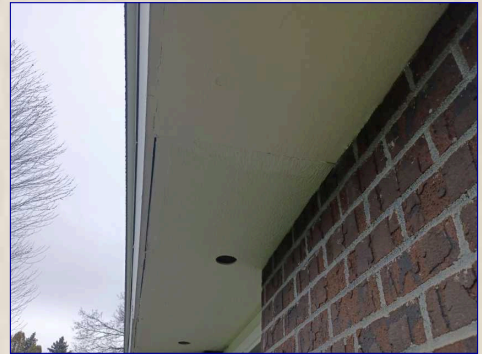
The soffit needed routine painting & maintenance.
