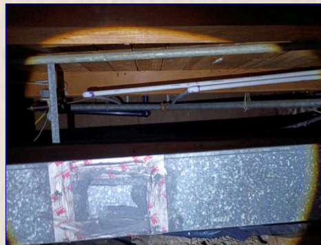
The visible water distribution piping.
