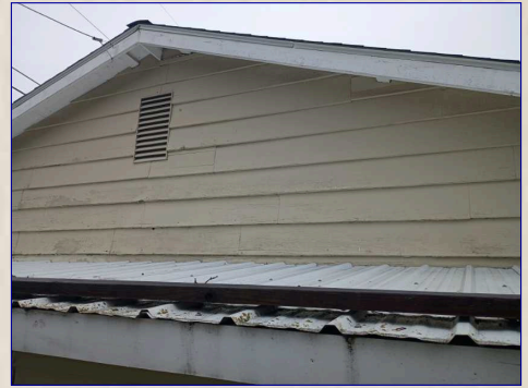
The siding needs routine repair and painting maintenance.
