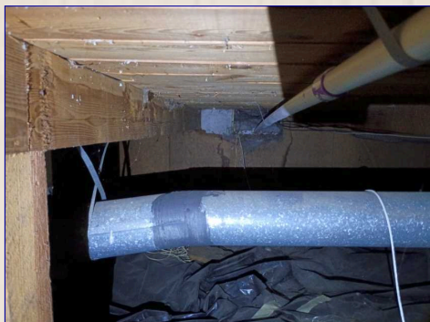
There are no wall vents in the crawl space area. Monitor and consult a licensed contractor as needed.
