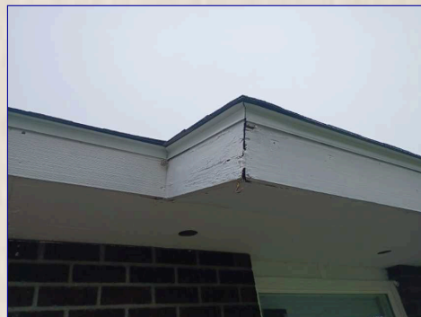
Fascia / Soffit needs maintenance
