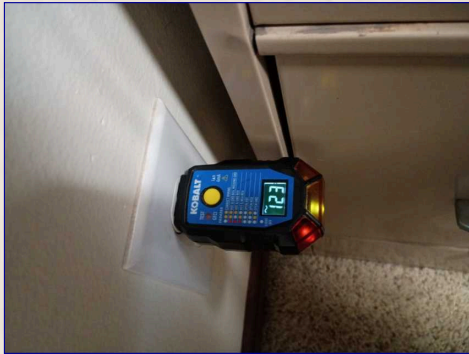
Electrical Receptacles in Bedroom 3 Wired incorrectly
