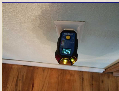
Electrical receptacle operating
