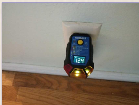
Electrical receptacle operating
