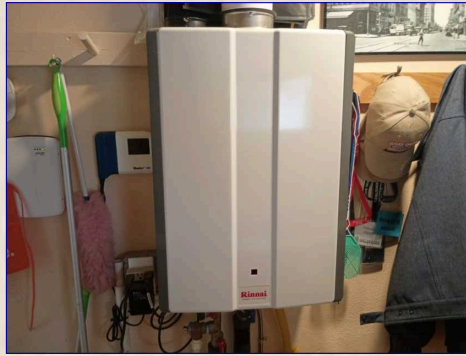
The Water Heater Area
