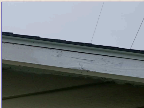
The fascia needs routine painting maintenance.
