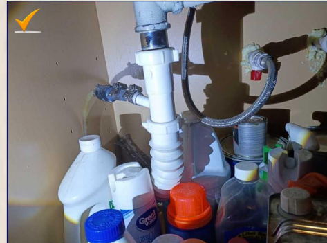
Laundry plumbing view.
