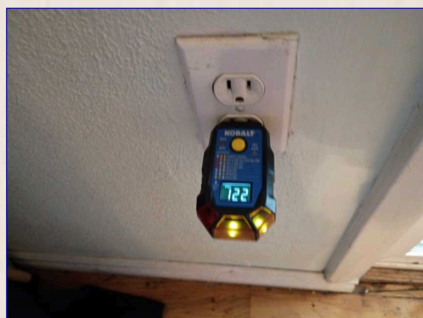
Electrical receptacle operating
